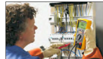
Insulation test at a distribution panel
