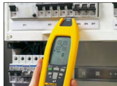
Location of fuses/breakers and assignment to circuits
