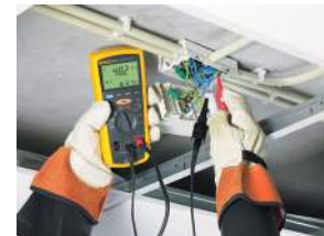
Wiring test in a small distribution box – all in one spot
